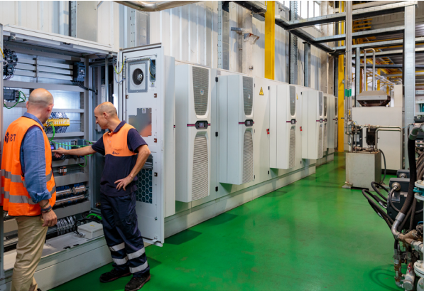
Secure remote access without causing production downtime is a must. Angel Ventura, Director of Engineering together with Javier Mallor, Head of Automation
