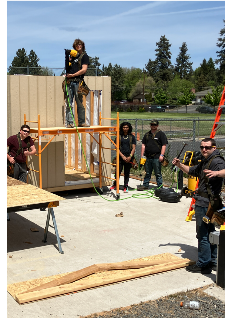
Bend Tech Academy students build emergency shelters following wildfire. Photo Credit: The School Foundation
