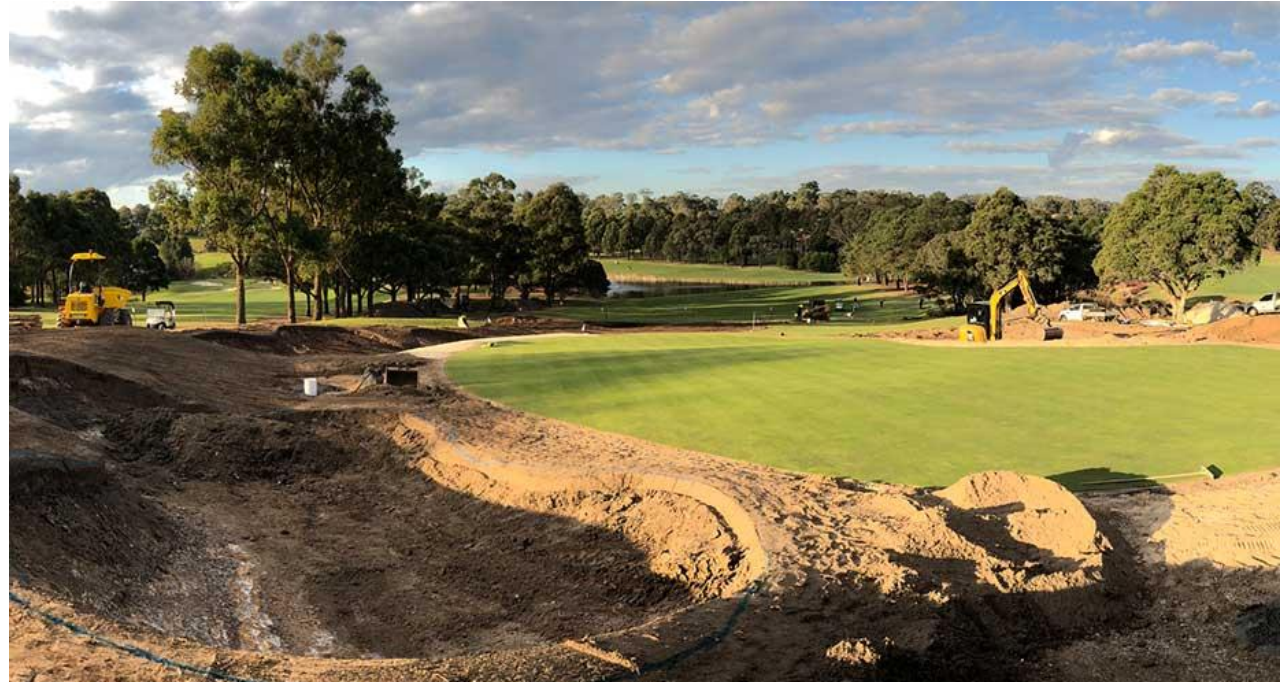
Construction underway at Castle Hill Golf Course in Sydney Source: Harrison Golf
