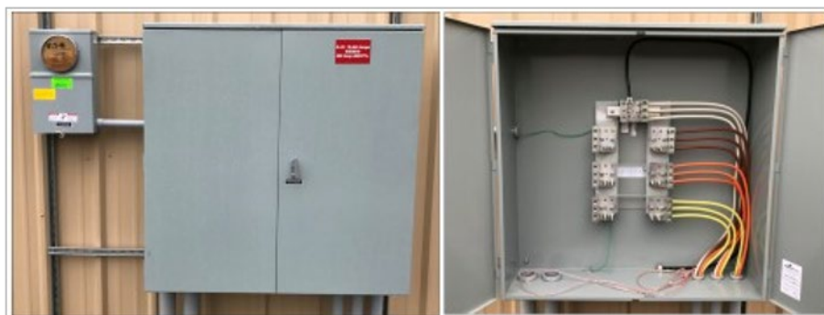
Figure 94. Typical Vertical Current Transformer Metering Installation
