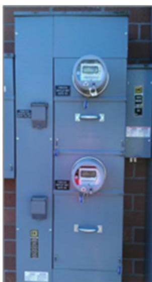
Figure 89. Typical Double-Stacked Module Meter Sockets
