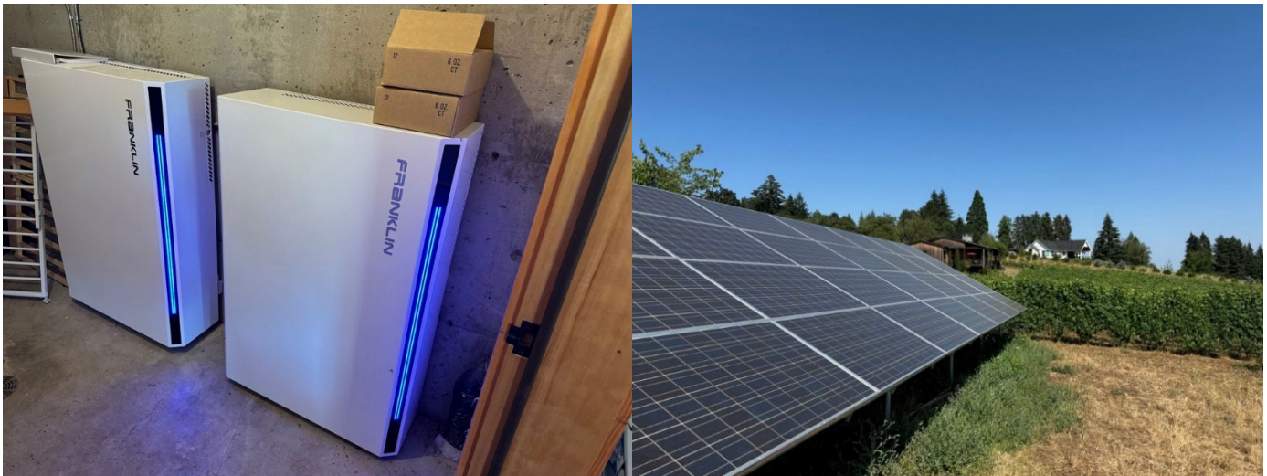
Figure 118: Battery Energy Storage and Solar for Well Water Backup
