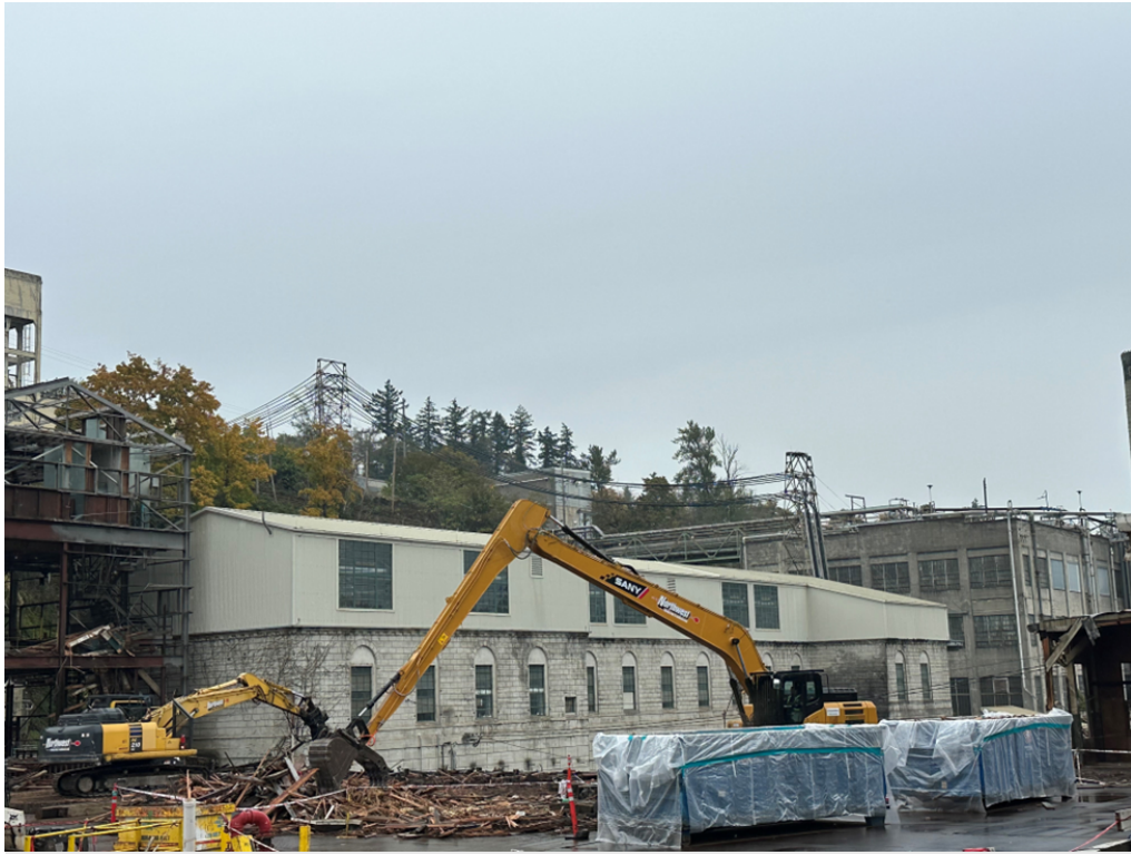
New views from the south of PGE's Sullivan plant
