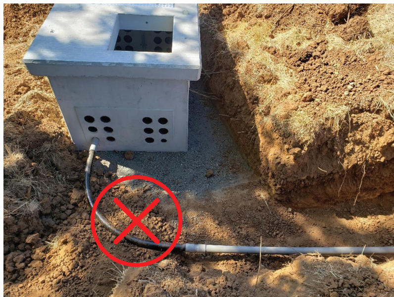
Figure 25. Conduit Exits Vault without Minimum Required Straight Section
