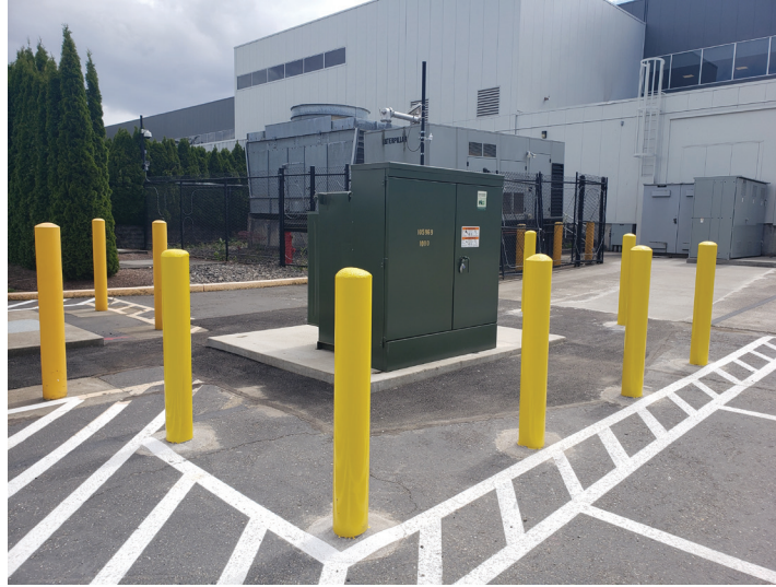
Figure 33. Barrier Post: PGE Equipment is Accessible to Vehicular Traffic
