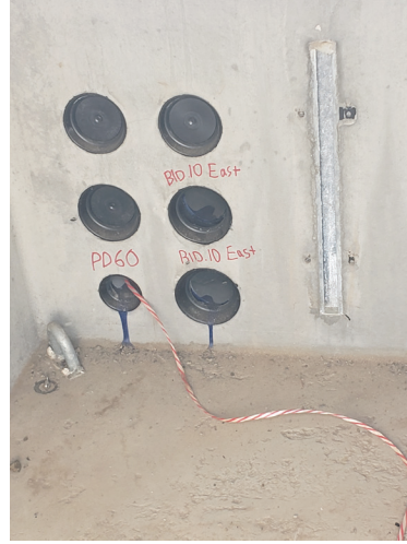
Right: Correctly installed ducts:
