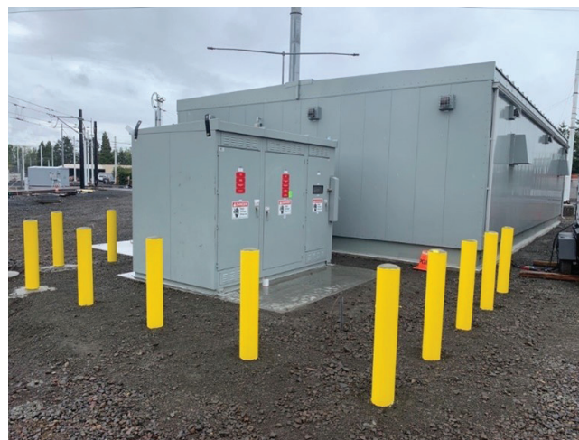
Figure 35. Barrier Post: PGE Equipment is Accessible to Vehicular Traffic
