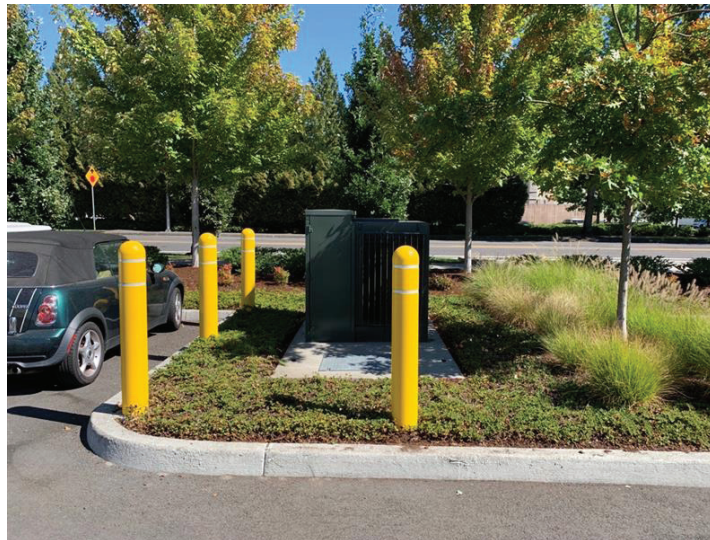
Figure 34. Barrier Post: Distance from the 6" Curb to the Pad is 5' or Less
