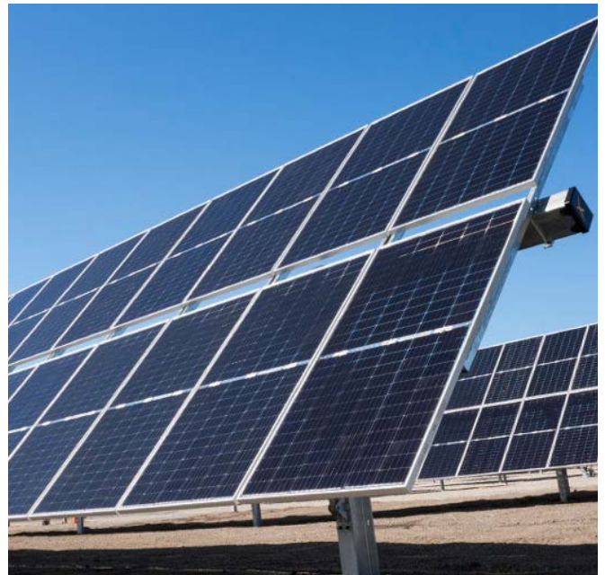
IMAGE OF A TRACKER SOLAR PANEL SYSTEM 4
