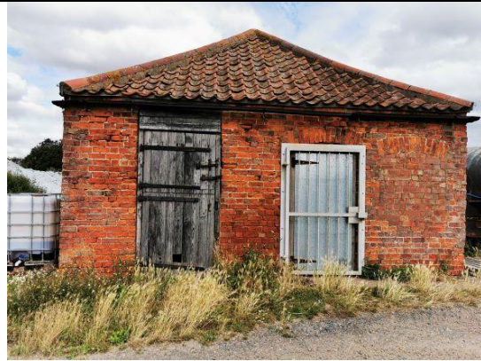
T8b – showing cracks in single storey cowshed from south offering low to medium bat roosting potential (BRP 3-2)
