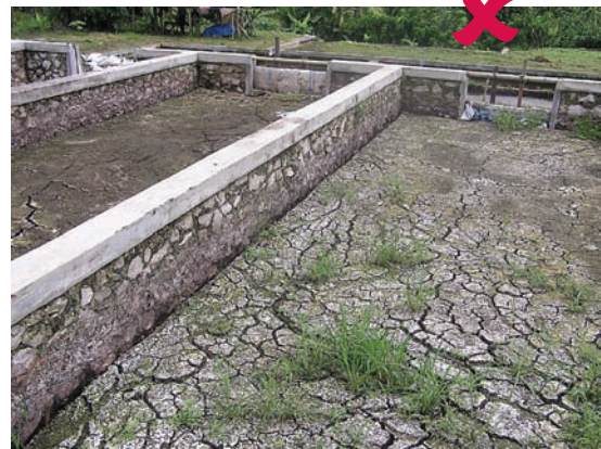
Sedimentation structure overdue for solids removal and stockpiling.
