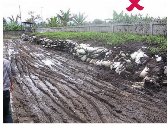
Uncovered stockpile causes bogging and creates contaminated runoff.
