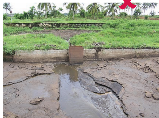
Poorly maintained sedimentation structures and choked overflows prevent good drainage.
