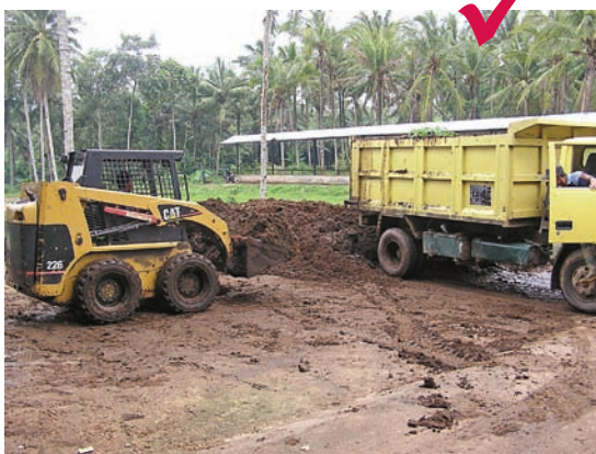
Solids cleaned from pens being loaded into a truck for transfer to stockpiles.
