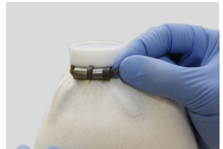
Isolate the corresponding areas of the objects that will be included in the laminate (e.g. screw heads, bare threads, joint surfaces) using the pre-formed Plastaband.
