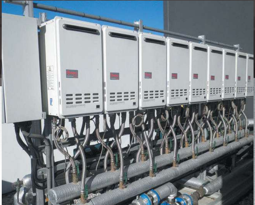
Photo: Back to back 18 Unit Commpak Plus®
