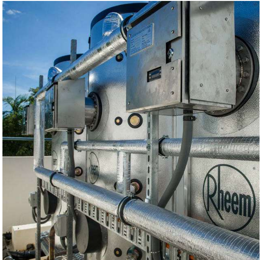
Rheem HS Series solar with electric boosting in the top of solar tanks. Katherine Hospital NT.
