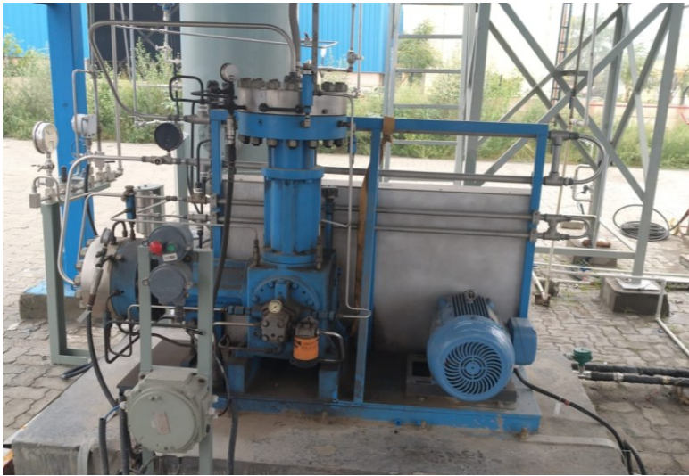
Fig. 8. Site photograph of the Diaphragm Compressor
