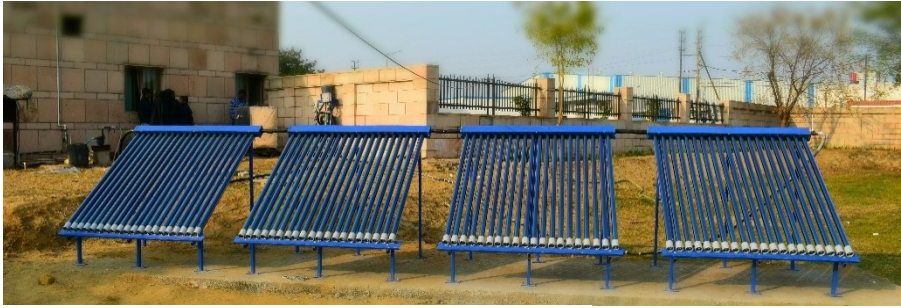
Fig. 5. Photograph of the Installed system.
