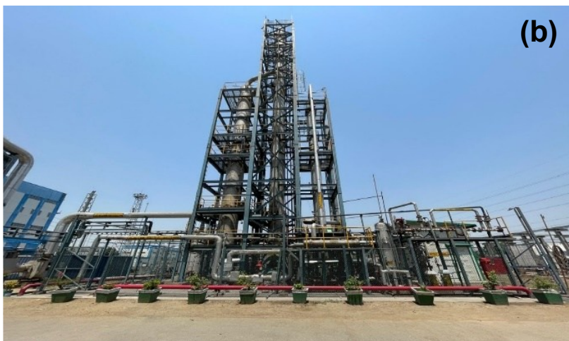
Fig. 1. (a) CO 2 Capture: Process flow diagram (b) Photograph of the CO 2 Capture pilot plant at NTPC Vindhyachal.
