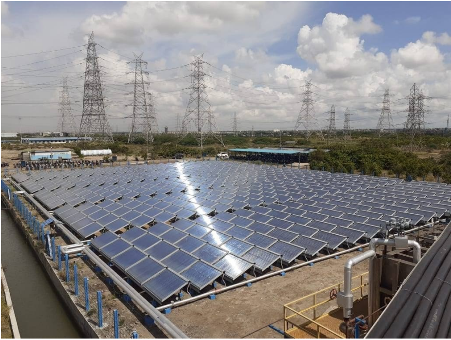
Fig. 6. Site photograph of the Solar Thermal (ETC-CPC) field of 2,420 m 2
