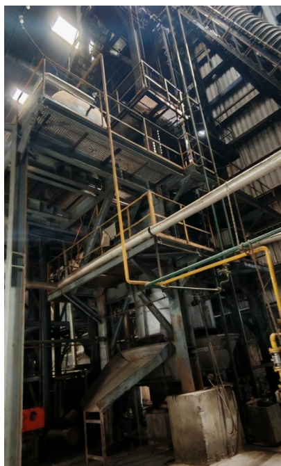
Fig.4. Photograph of the MSW/RDF Gasifier
