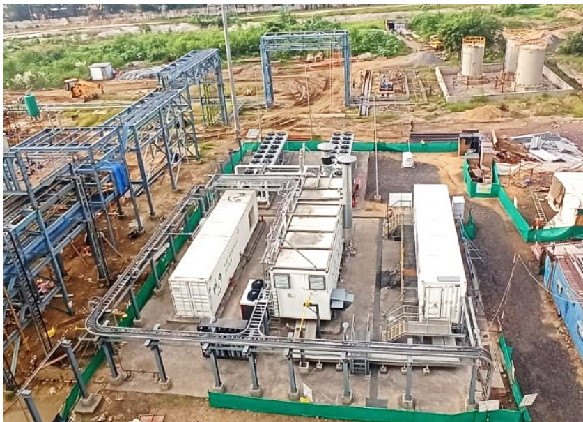
Fig. 2. Photograph of the PEM electrolyzer installed at NTPC Vindhyachal.
