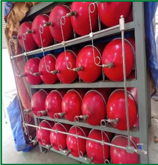
Fig. 9. Site photograph of the Hydrogen Storage.
