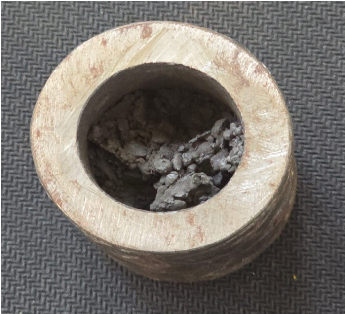
Fig.1. The picture showing boiler tube blockage with predominantly iron and silica rich deposit.
