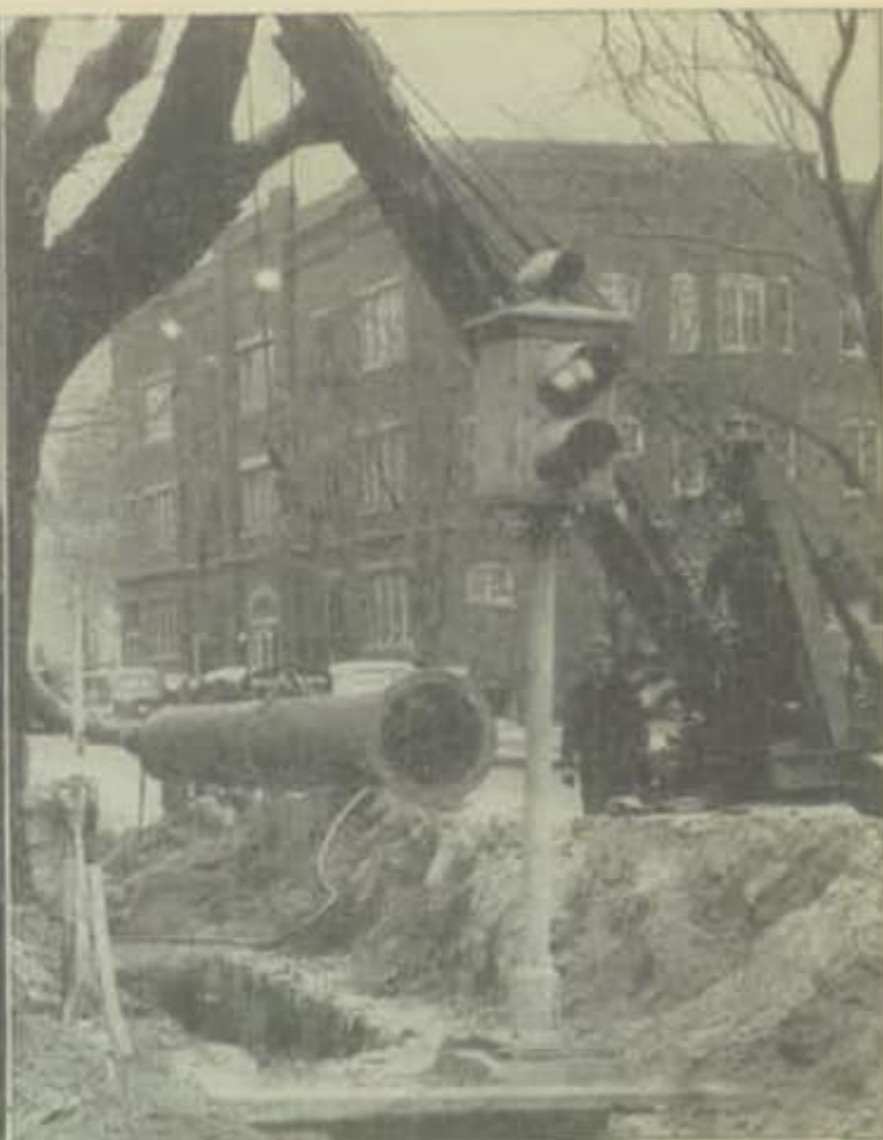
Kenosha, Wis. Removing a 14-inch cast iron water main for replacement with new 24-inch cast iron pipe. After 43 years' service, the old 14-inch pipe proved to be in excellent condition and was relaid in another section of the city.
