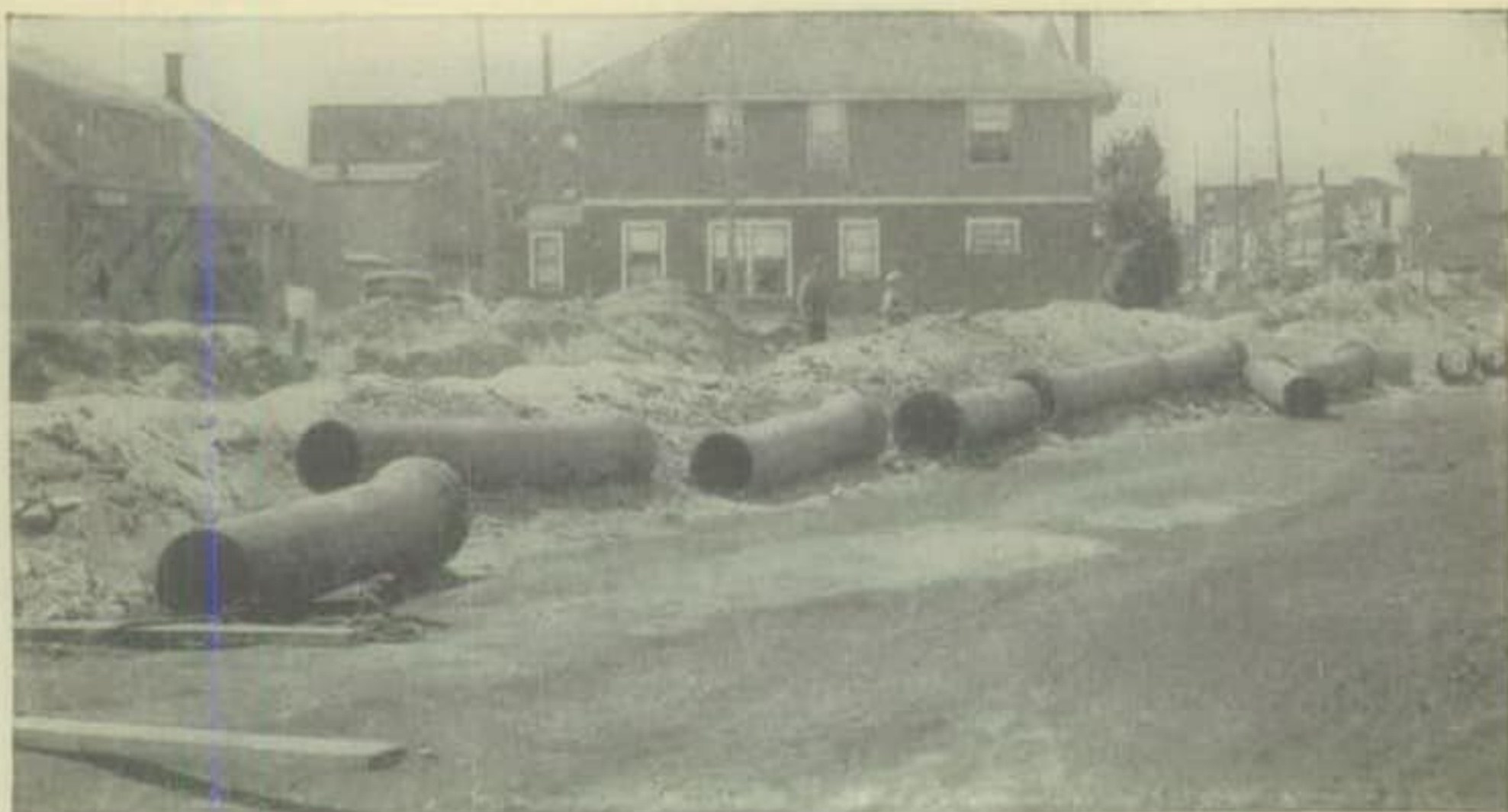
Escanaba, Mich. This 16-inch cast iron pipe, after nearly half a century of service in the water supply system of Iron Mountain, Michigan, was taken up and relaid in Escanaba, about fifty miles away.
