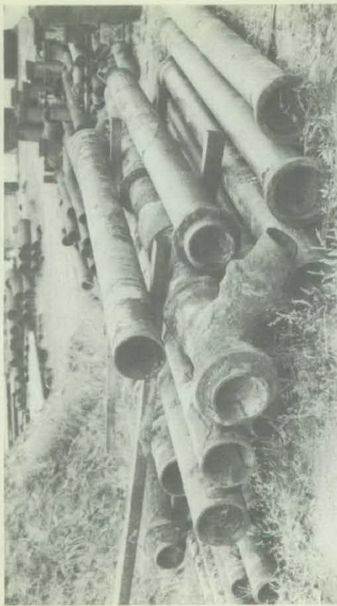
TRAVERSE CITY, MICHIGAN—"Pipe was just as good after 65 years of service as when it was put into the ground." This is the report issued on this 8-inch cast iron pipe which was removed for replacement of larger diameter cast iron pipe. Future plans for this pipe: re-use wherever it can be installed in the system.
