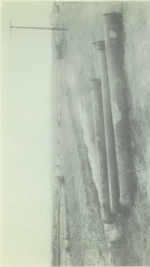
CHARLESTON, SOUTH CAROLINA—Tidewater area conditions didn't phase this 16-inch gravity outfall line for cast iron pipeline installed in 1944. New Interstate highway interchange required new location of line which was completely submerged at high tide. Condition of this pipe was remarkably good after 17 years' exposure under these tough conditions.
