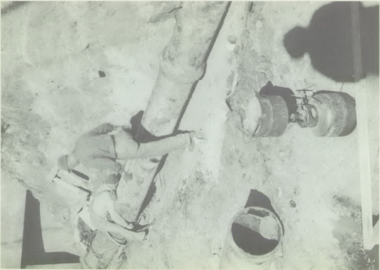
FERGUS FALLS, MINNESOTA—New water plant uses 50-year-old pipe. That's the history of this cast iron pipe installed originally in 1916 and salvaged and re-used nearly 50 years later. Pipe report: "excellent condition."
