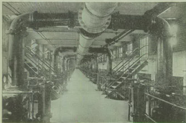
Cast Iron Pipe in the Filter Gallery
