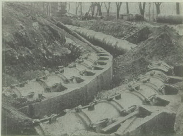
Lugged Bends Reinforced with Masonry Piers
