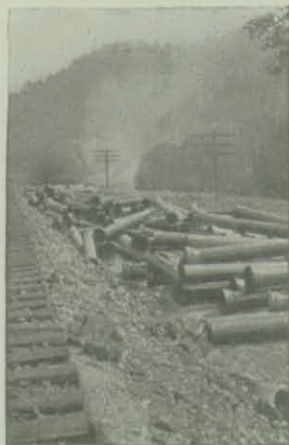
Pipe Improperly Unloaded
