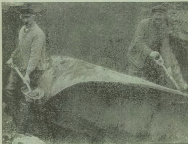
Large Rock Directly Under Break in Pipe
