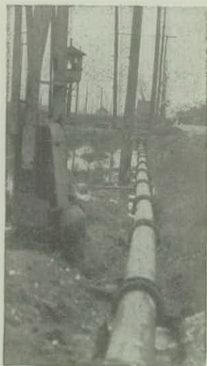
Dresser Type Couplings on Small Pipe
