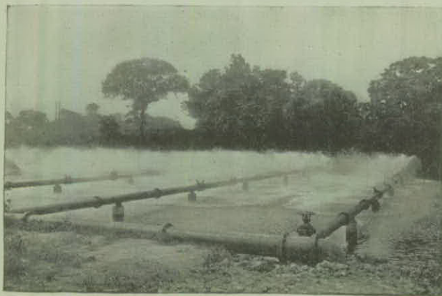
Spray Cooling Pond Piping
