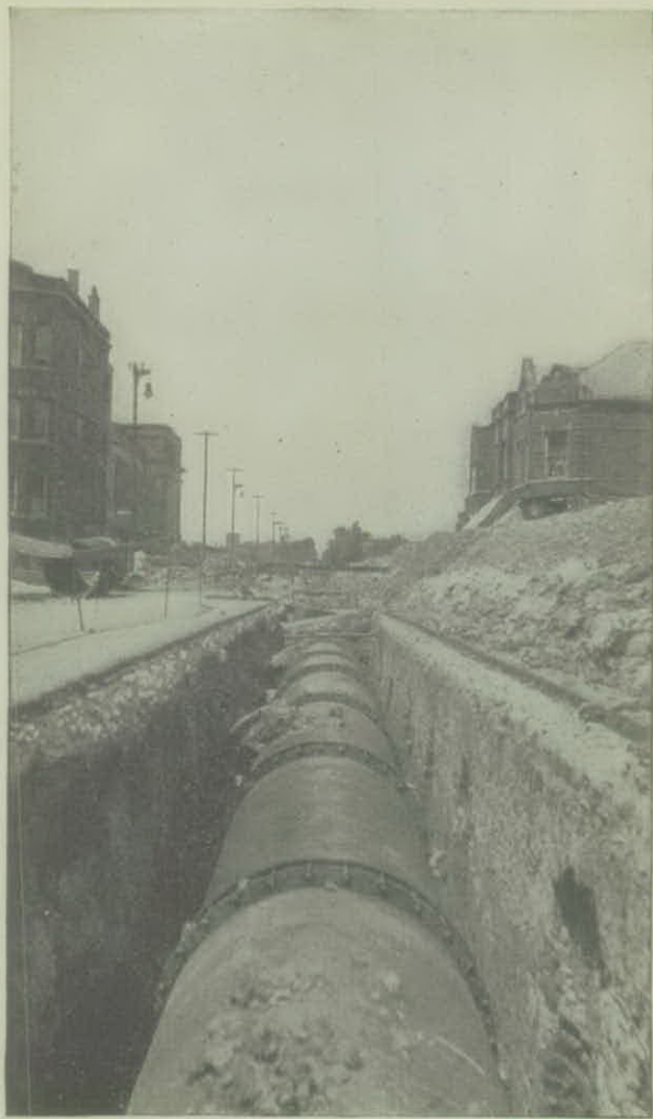
48-inch Plain End Gas Pipe with Dresser Couplings
