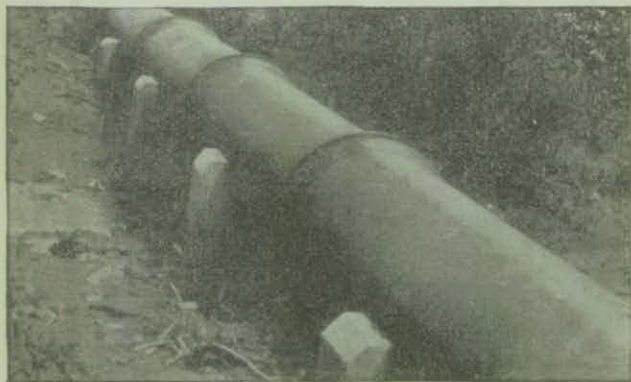
Pipe Supported on Concrete Piers
