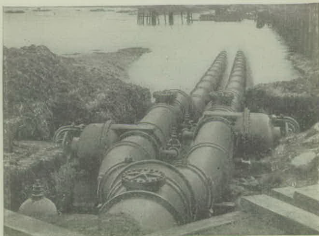
Two 36-inch Submerged Water Lines with Valve Connections
