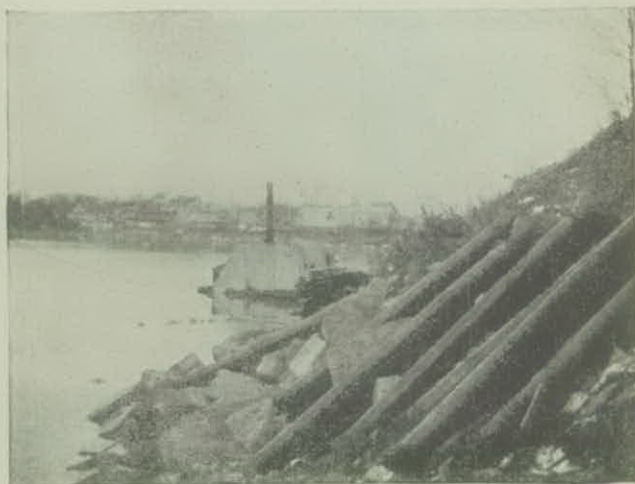
Careless Unloading Resulting in Serious Damage to Pipe
