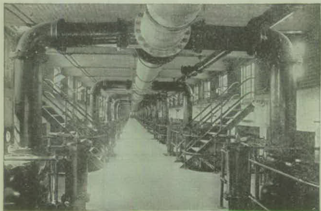
Cast Iron Pipe in the Filter Gallery
