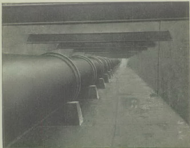
Large Sewer Siphon Line
