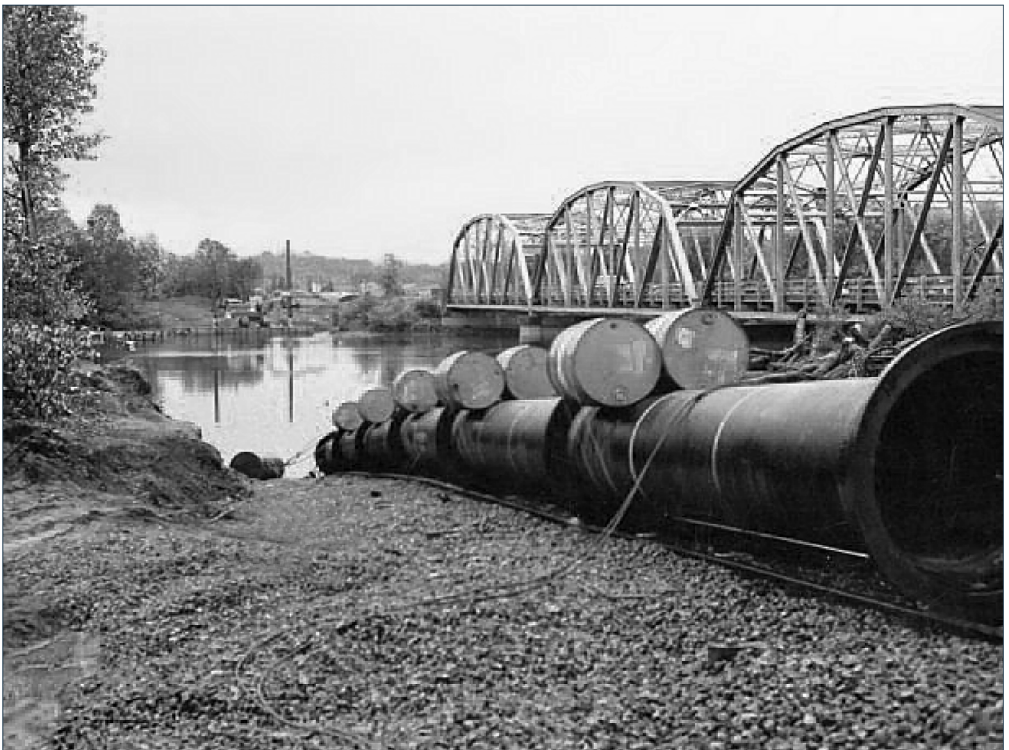
For some pipe sizes, it is necessary to provide additional buoyancy to float the pipe into position. Here, steel drums are used for that purpose.
