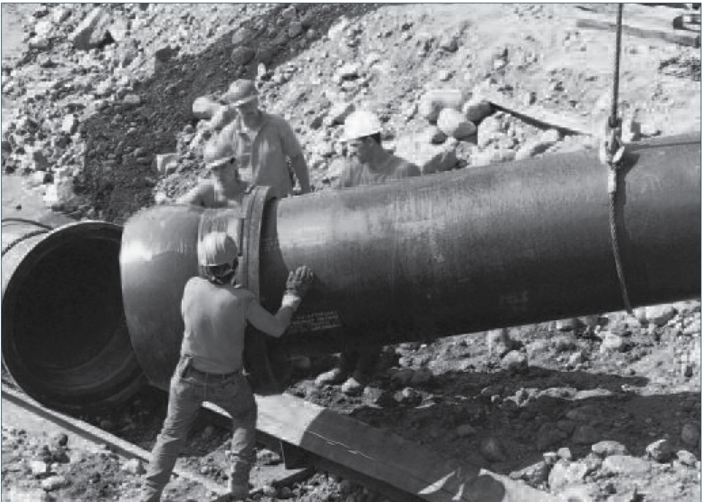
In many subaqueous installations, the majority of the assembly can be done on dry land. Here, a crew lowers a piece of Ductile Iron Pipe into place on top of a launching ramp from which cables will pull it across the water.
