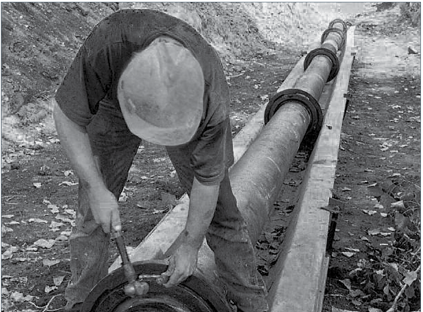
Finishing assembly touches are made to a Ductile Iron Pipe joint. This particular pipeline is cradled in an inclined launching ramp that prevents the pipe from touching the ground. This facilitates clean joints and will make it easier and faster to pull the pipeline across the water.
