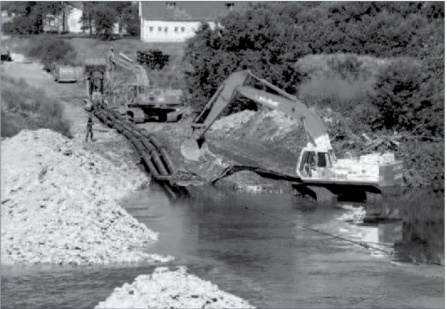
Portions of three parallel pipelines assembled on land are shown prior to their being pulled across the water. Ductile Iron Pipe's durability and deflection capabilities make it ideal for installations in this situation as well as other rugged water crossings.
