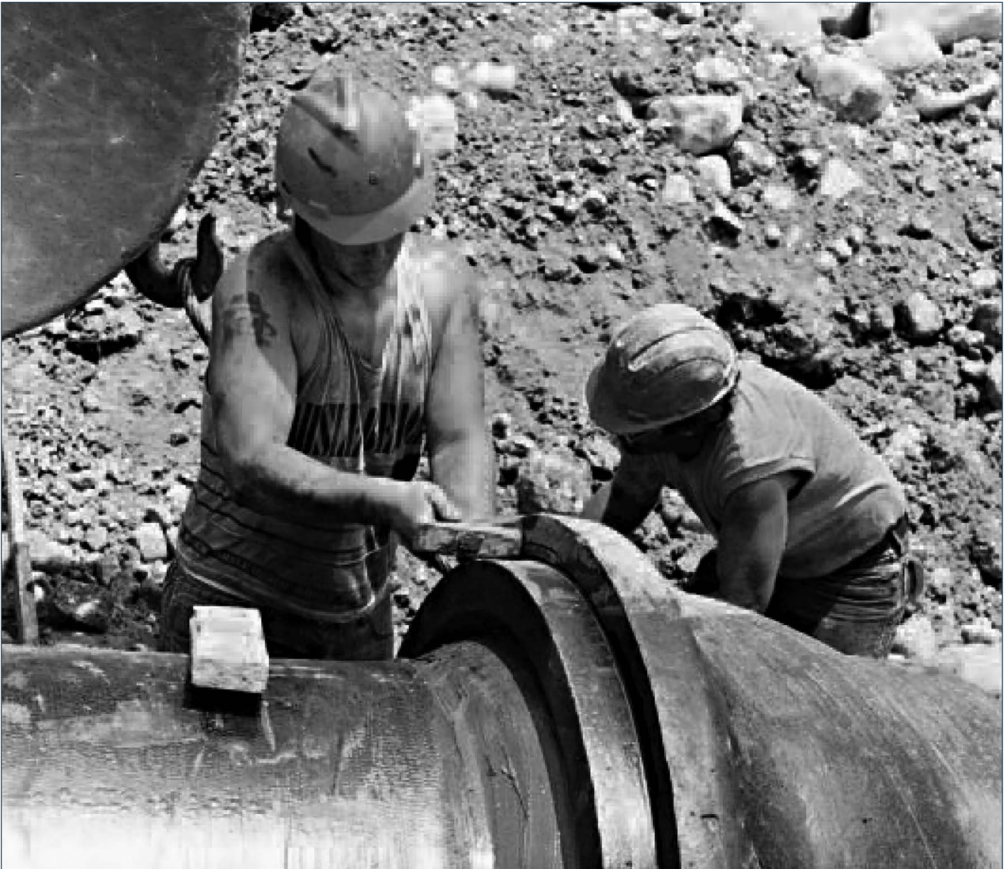
An installation crew member is shown driving a steel wedge into a pipeline joint. The wedge provides a lock that prevents rotation of the locking gland after assembly.
