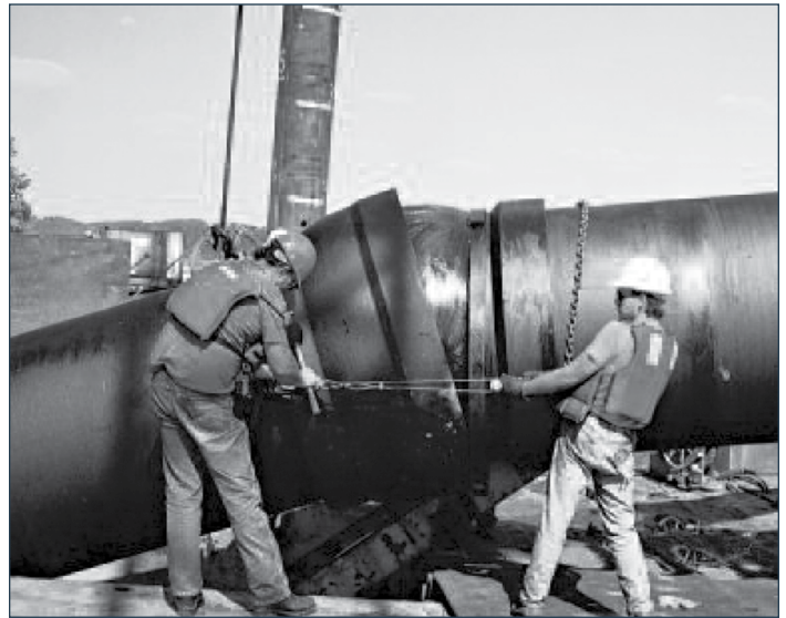
Workers use come-alongs while installing Ductile Iron Pipe with boltless ball and socket joints. These joints consist of a precision-machined ball that fits into a precision-machined socket, a rubber gasket that provides a pressure-tight seal, and a retainer ring that provides longitudinal restraint. The joint is leak-free throughout the full range of deflection.
