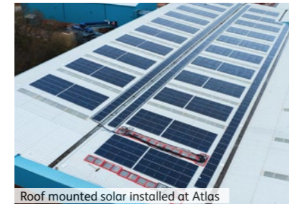
Roof mounted solar installed at Atlas
