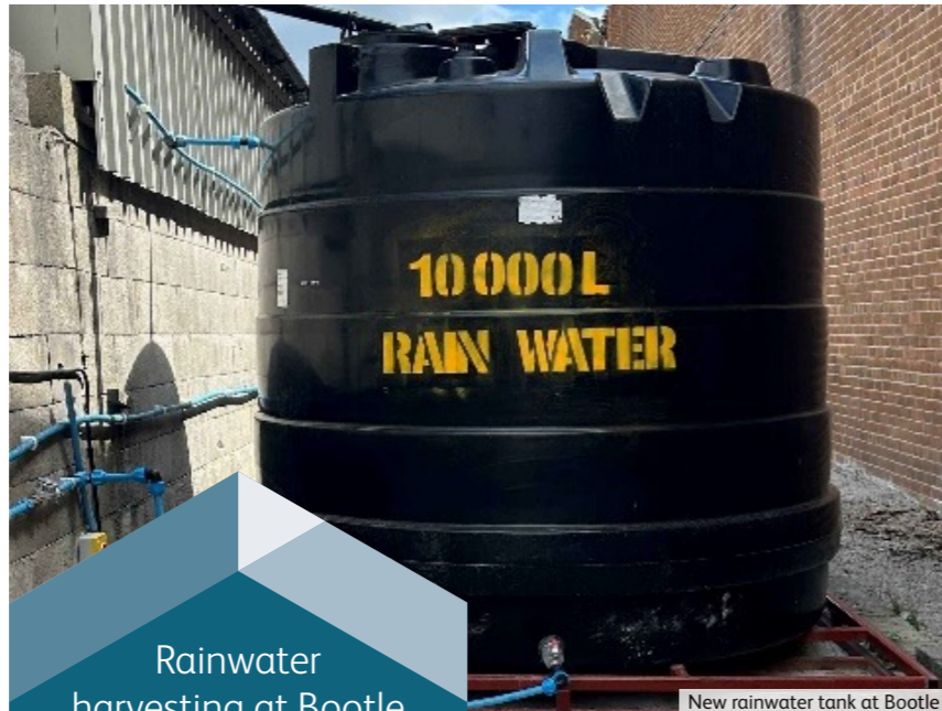
New rainwater tank at Bootle
