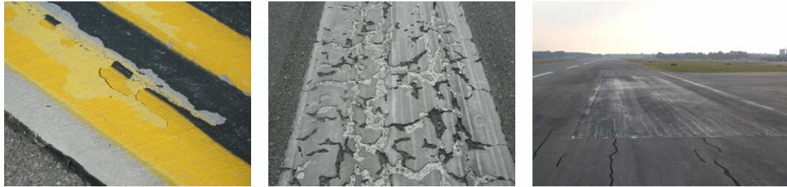
Figure 12.1: Examples of Deteriorated Pavement Markings
