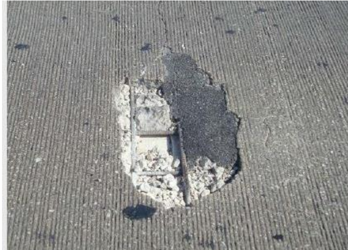
Figure 9.17 Damaged Bridge Deck
