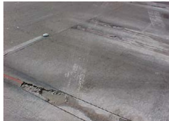
Figure 1: Crack and Spall
