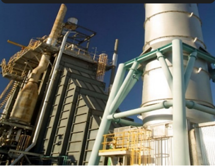
MICA CREEK POWER STATION
