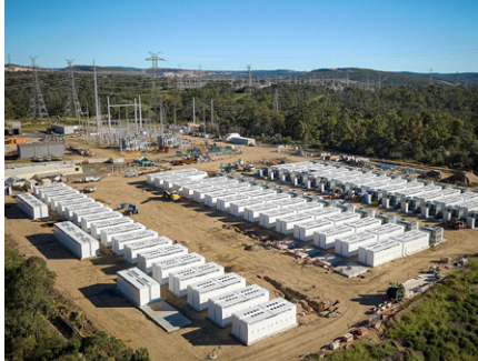
CENTRAL REZ BATTERY
