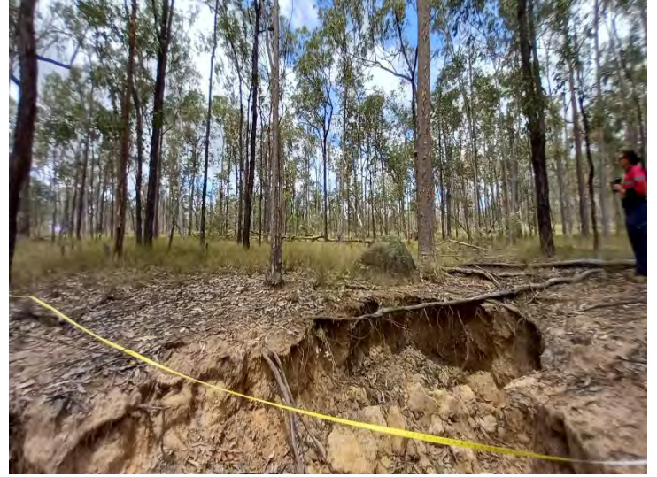
Plate 2 Erosion 1 east view.
