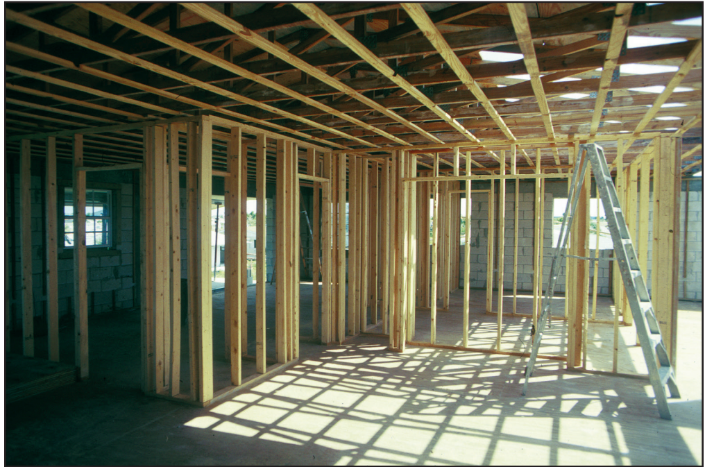
Figure 48 Wood 2 by 4 studs were used to frame the interior walls of the second story.
