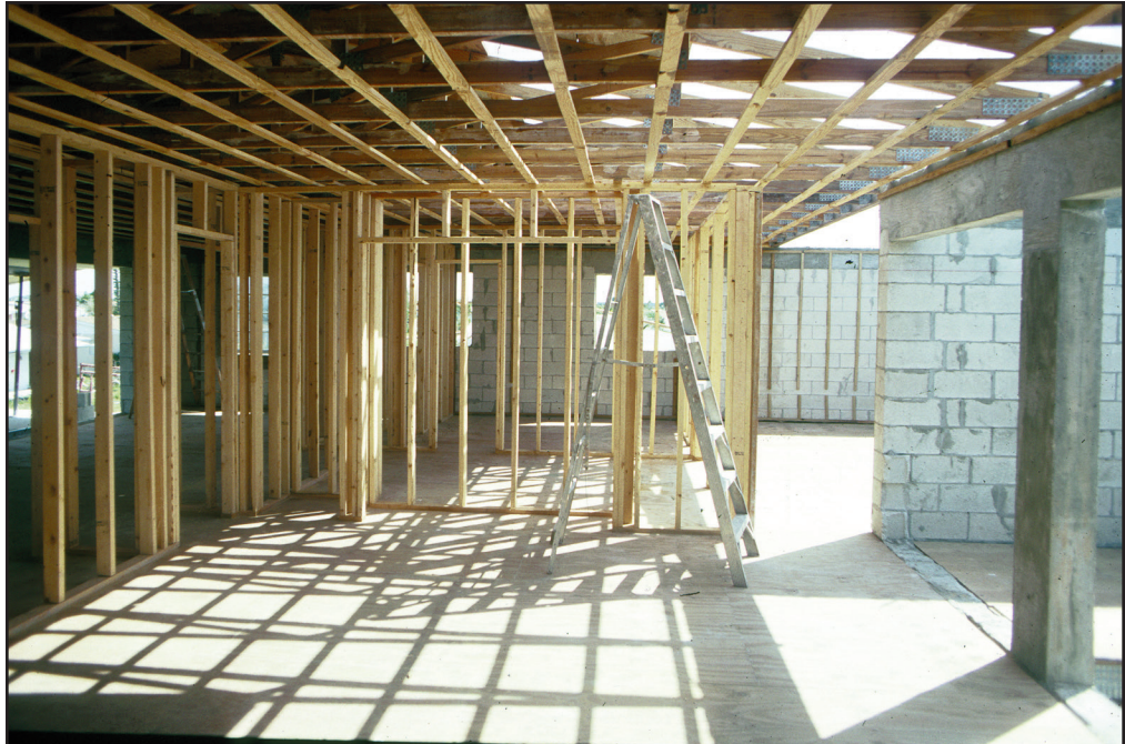
Figure 34 After the new concrete slab is poured, wood framing for interior walls is added.
