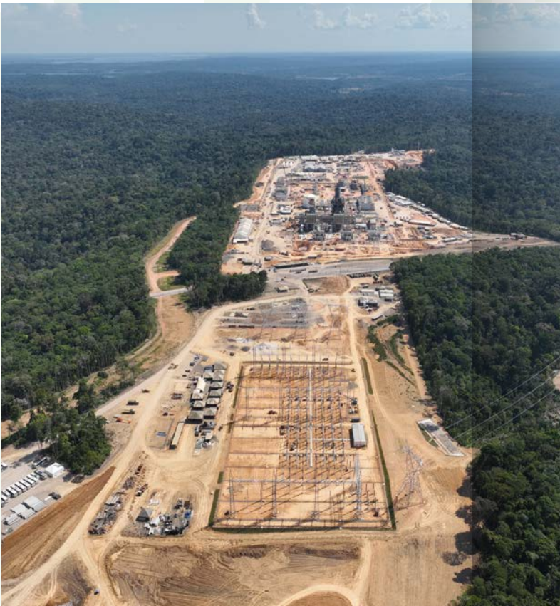
ENEVA Manaus - Brazil Implementation of an integrated telecommunications system for the development of the Azulão onshore gas field: CCTV, access control, radar intrusion detection, fiber optic network, switches, firewalls, IP telephony, telecom tower and communication infrastructure. By Ekium
