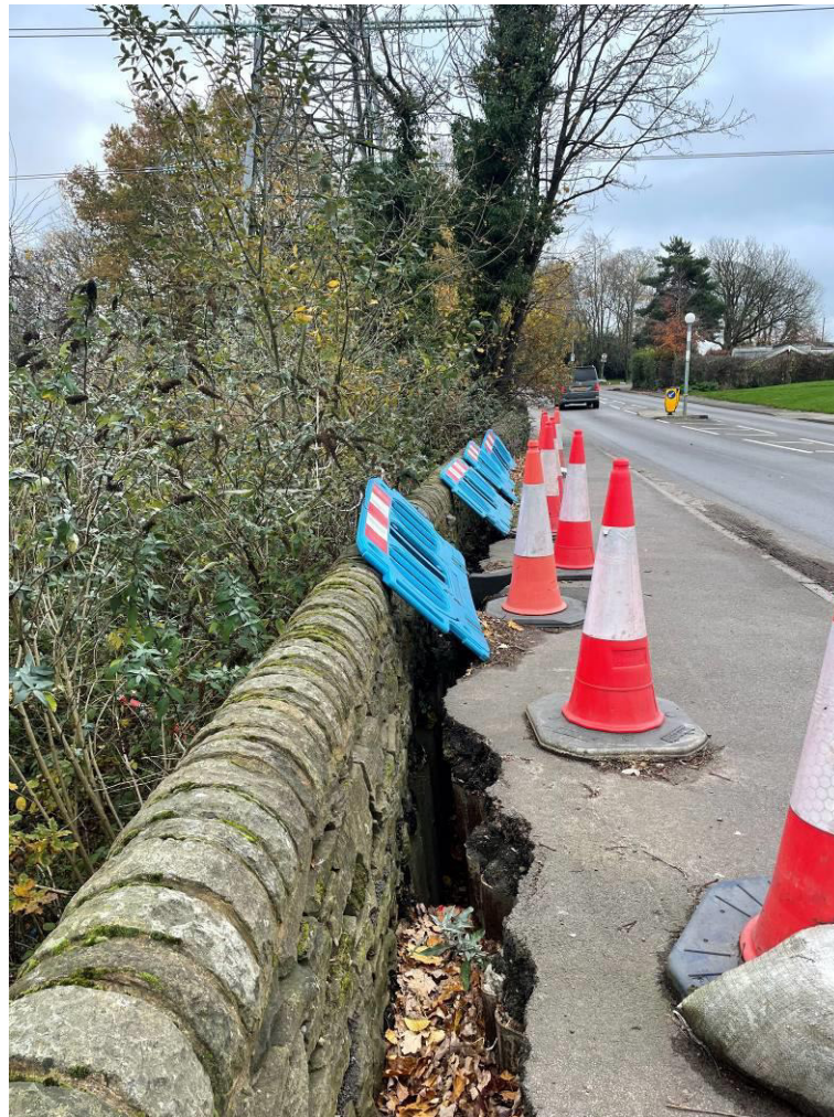
Gap between back of footway and stone masonry parapet, January 2023
