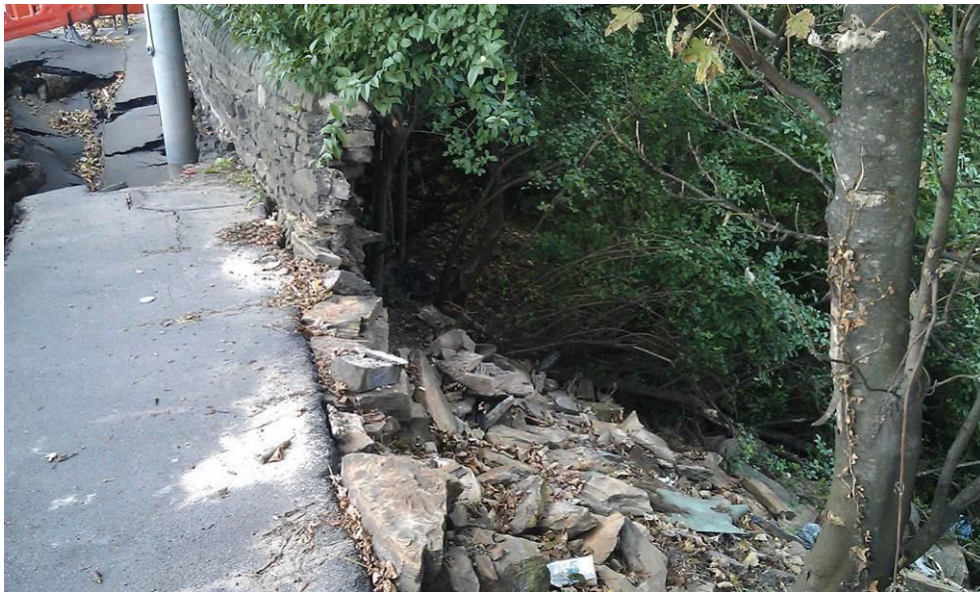
Photo of damaged footway / retaining wall circa 2013, prior to the commencement of works (provided by SMBC)
