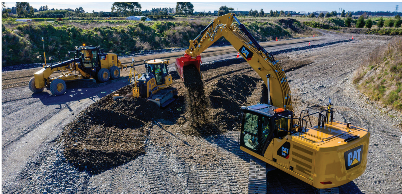
Construction is a highly fractured activity but by using digital workflows to link the various departments, contractors can enjoy increased efficiencies and better-informed decision making.
