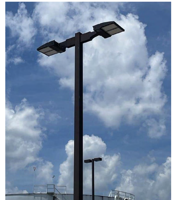
Pictured: LED lighting fixtures in the Fuel Farm parking lot
