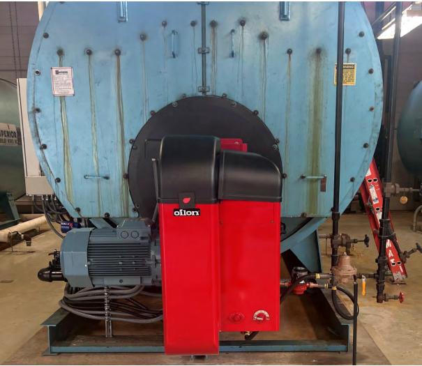
Pictured above is the new boiler at the Central Energy Plant.
