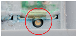
A contaminated main battery connector
