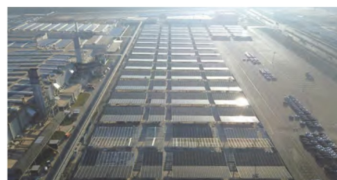
Photovoltaic canopies at a parking lot for FAW-Toyota commodity vehicles
