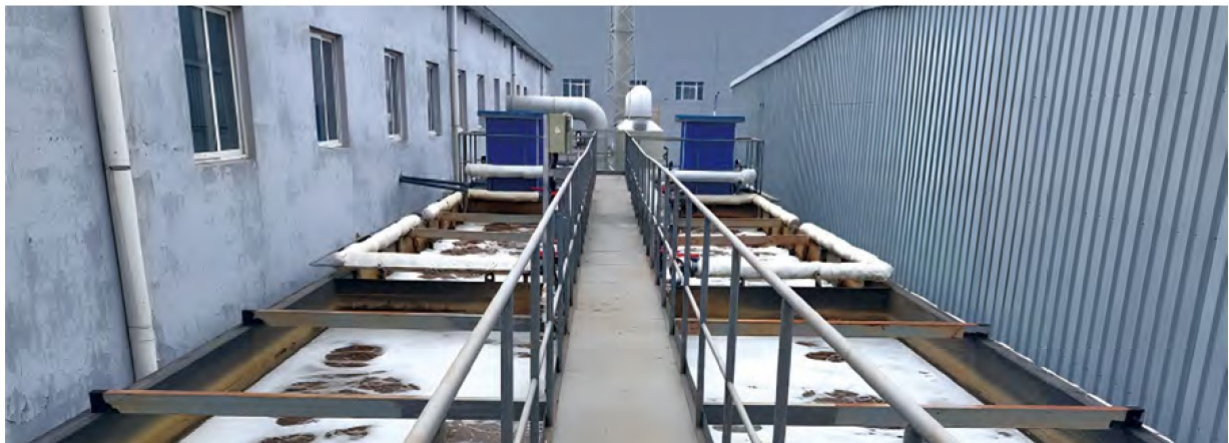
The MBR Re-Upgrading Project
