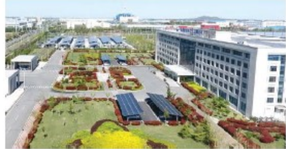
8.75MW distributed photovoltaic power generation project in the FAW Jiefang Qingdao Jimo Factory
