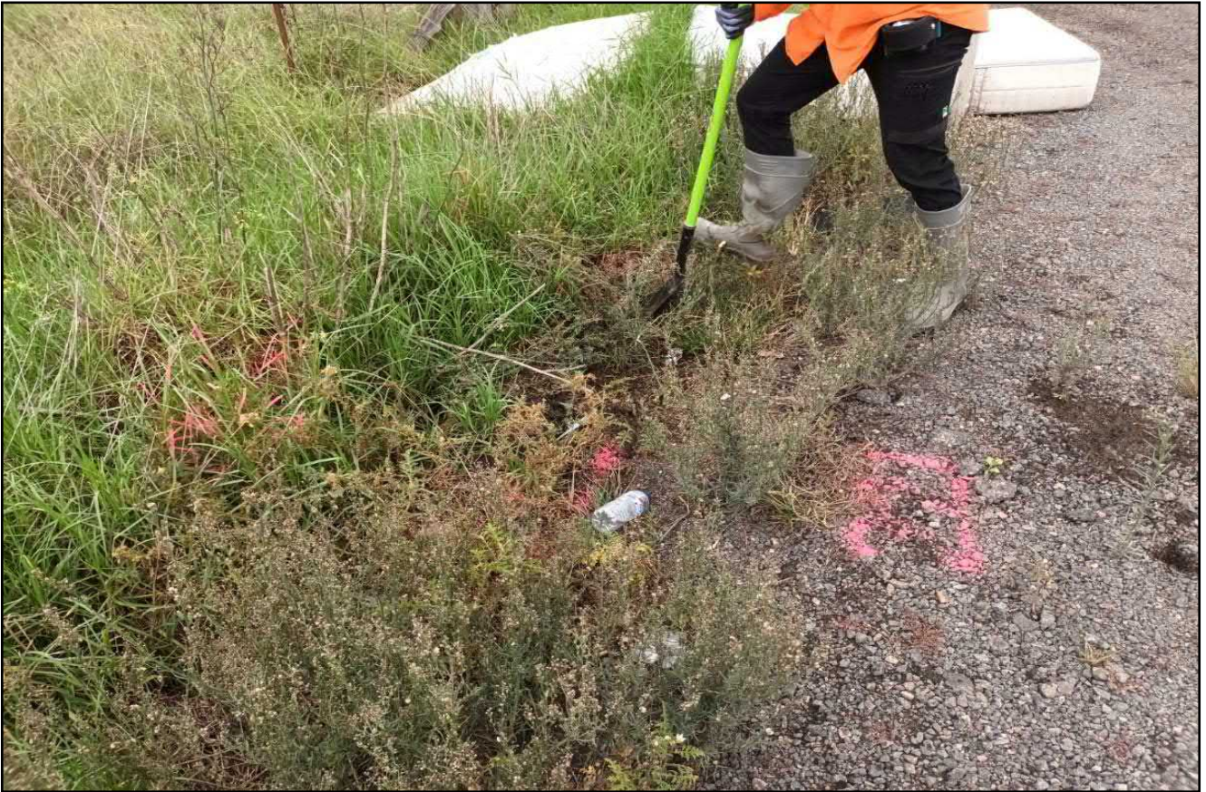
Photograph 13. Representative image of overgrown weeds adjacent to roadside which limited excavator access for safety reasons, at TP 223. Date: 28.03.2023.
