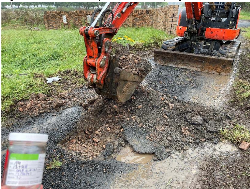
Image 8.1.1.1 Excavator used for all test pits at the location of DR11, facing west.
