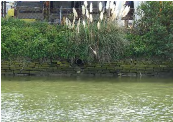
Figure 6. Stormwater outlet adjacent to 28 Burrows Road, view from the eastern bank (Source: LOGOS, 2022)
