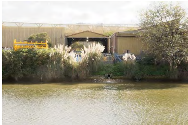
Figure 7. Canal wall adjacent to 30 Burrows Road, showing another storm water outlet, which has been releasing acidic drainage indicated by the lack of algae. (Source: LOGOS, 2022)
