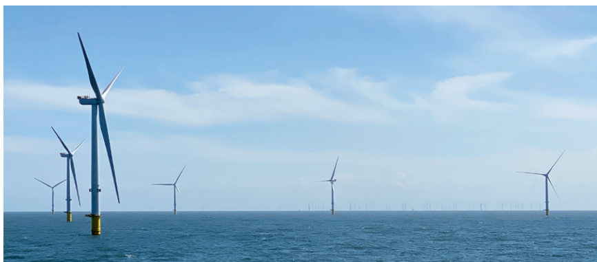
Above: Triton Knoll wind farm began turbine installation and achieved first generation in 2021.
