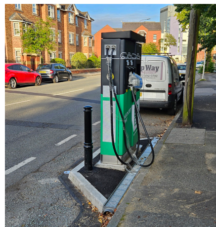
On-street EV charging facilities.
