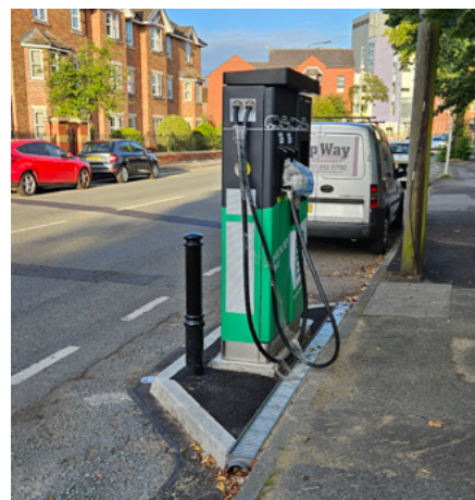
On-street EV charging facilities.
