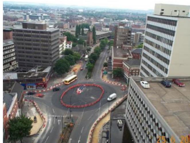
The selected design involved completely filling the subways and sunken plaza with concrete. Credit: Nottingham City Council
