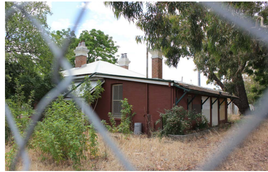
Boarded element to the east elevation. Source: SCA 12/12/2018
