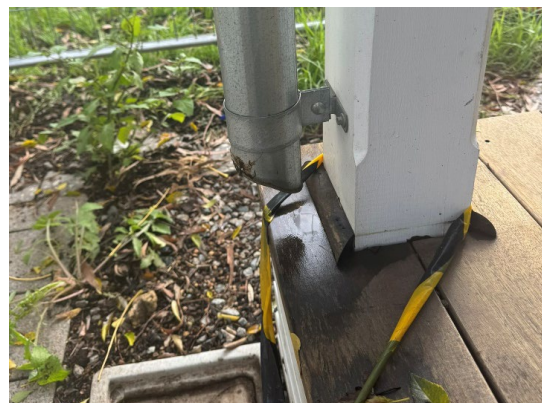
Figure 7 :Existing condition of west verandah rainwater goods. The foot of this DP is missing and disconnected from the drain.
