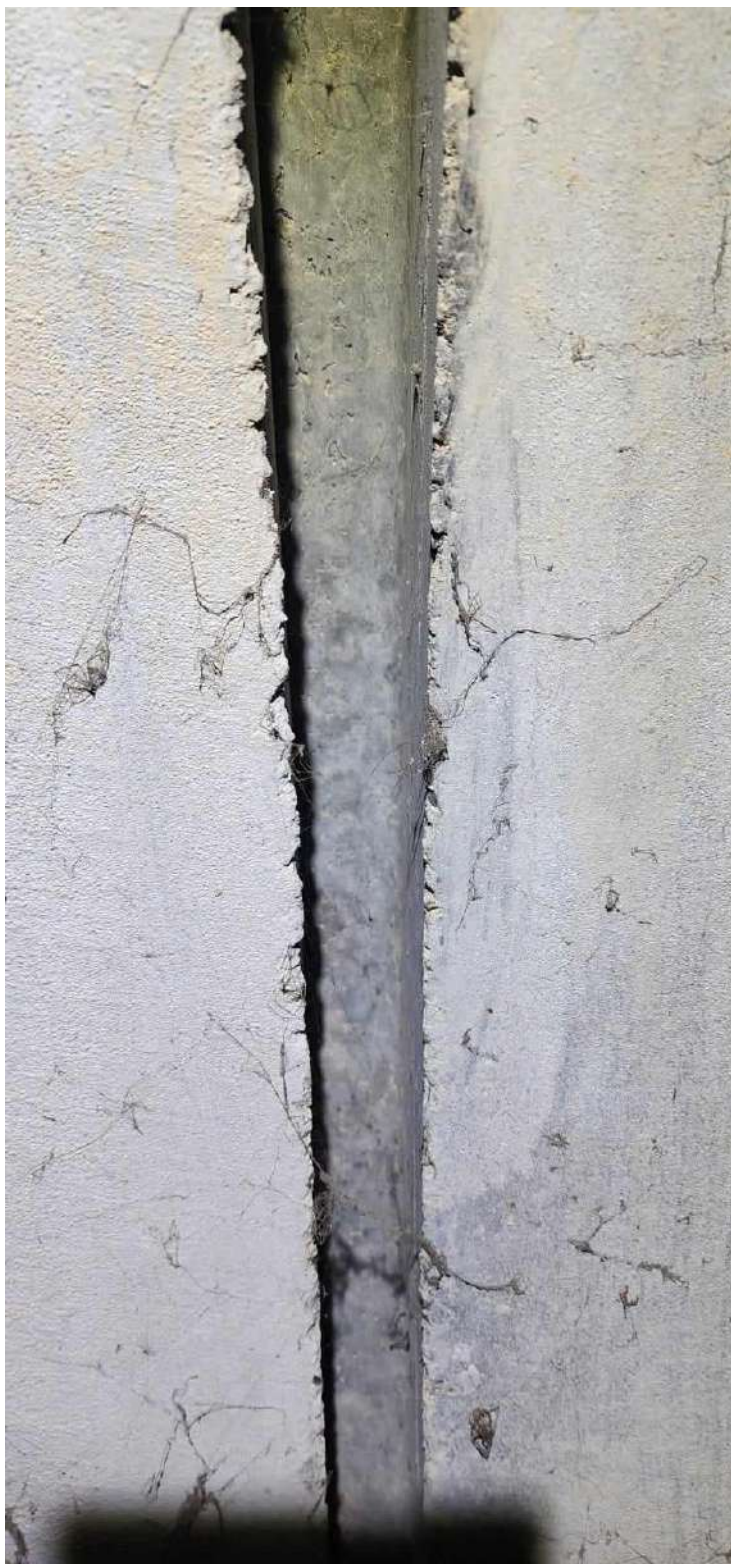
Figure 2. One of many cracks formed by the joins in the culvert sections. These cracks and other crevices were searched by torchlight during surveys. No evidence of Microbat presence was found.
