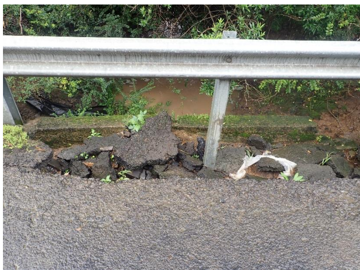
Figure 22. Broader of Survey Unit 1 and 2, view north showing drainage channel and broken road
