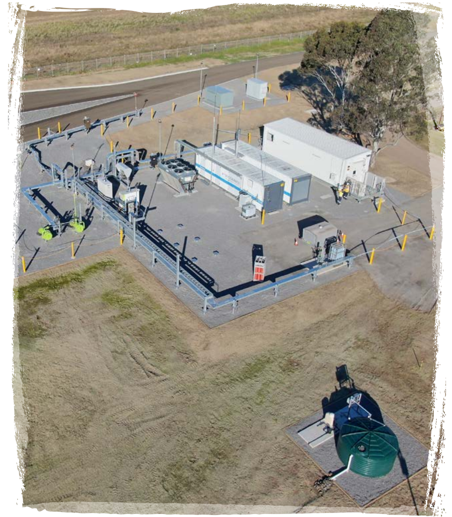
Our Western Sydney Green Hydrogen Hub is one of our Renewable Gas demonstration projects, operating since November 2021
