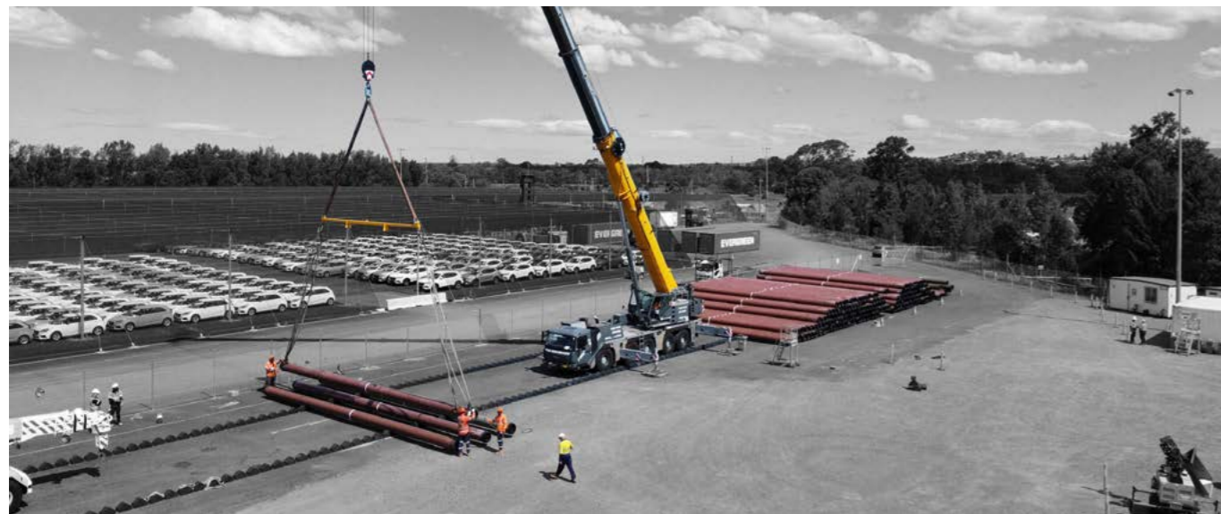
Construction for the lateral connecting the Port Kembla Energy Terminal to the Eastern Gas Pipeline was completed in 2024
