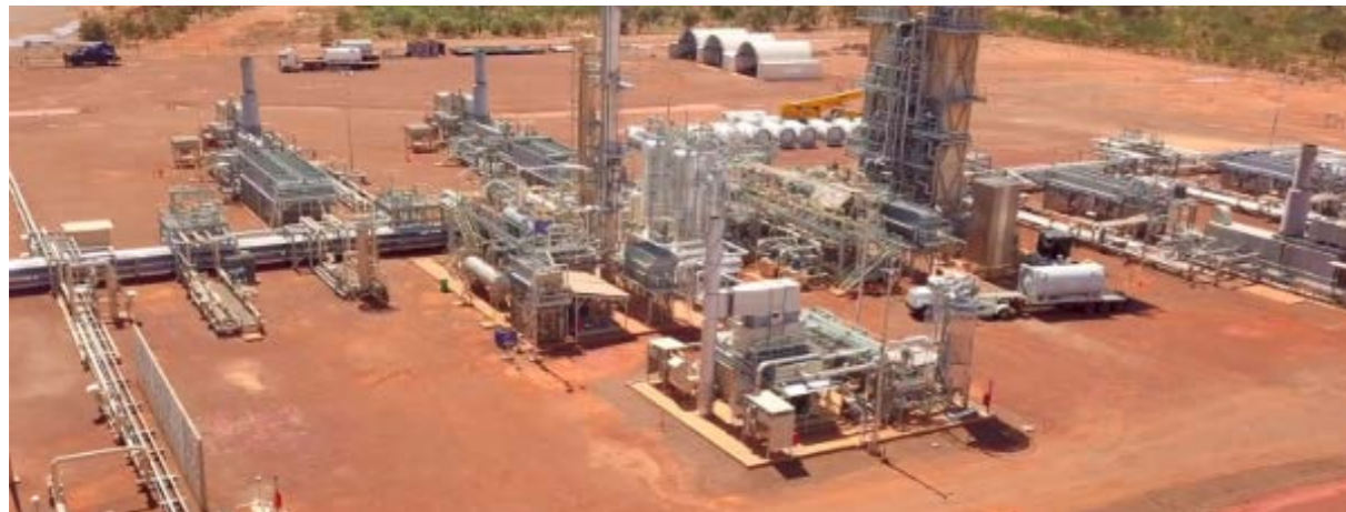
The Phillip Creek Compressor station
