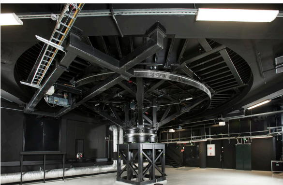
Stage gantries with equipment
