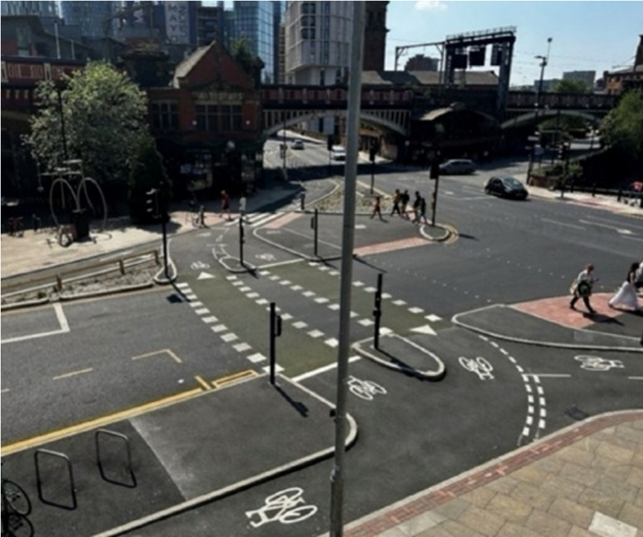
Figure 0-8 – Protected junction installed at the busy intersection of Deansgate/Whitworth Street in spring 2025
