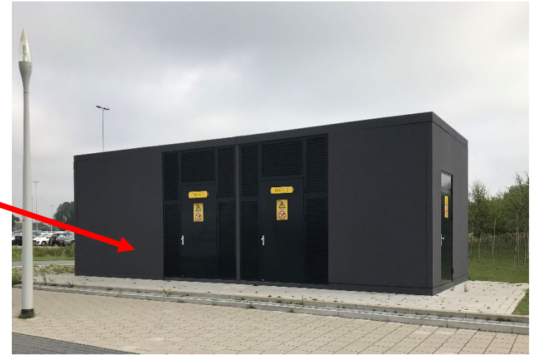
2 x > 900 kVA Transformers Independent for resilience
