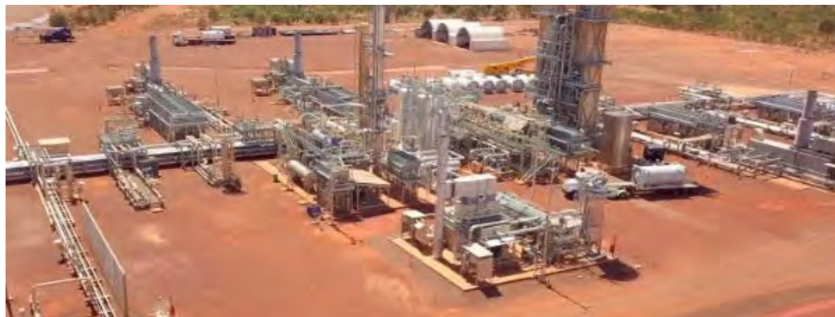
The Phillip Creek Compressor station
