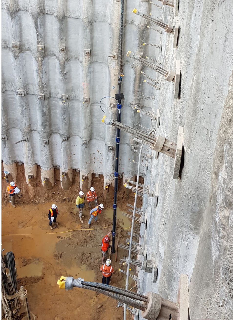
AUSTRALIAN CATHOLIC UNIVERSITY, ST TERESA OF KOLKATA BUILDING DYWIDAG DCP THREADBAR MICROPILES
