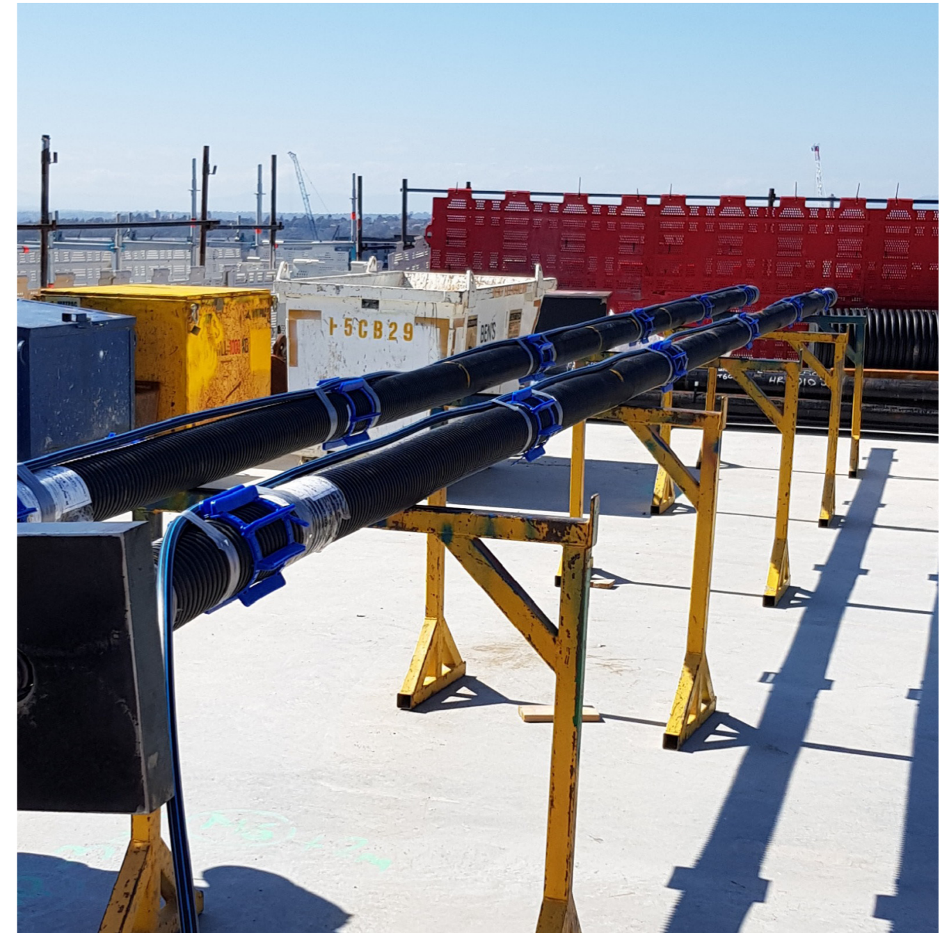
DOUBLE CORROSION MICROPILES
