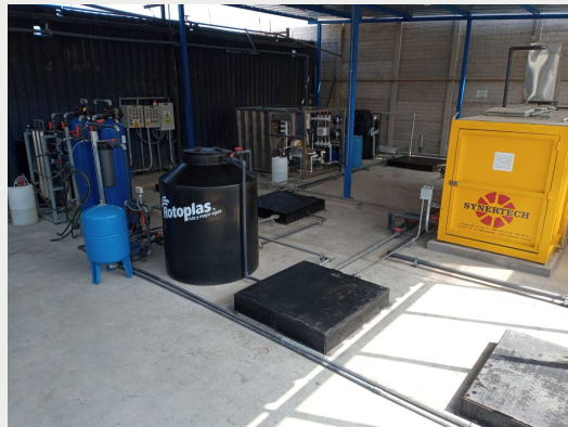
Water treatment plant in Villa El Salvador (Peru)
